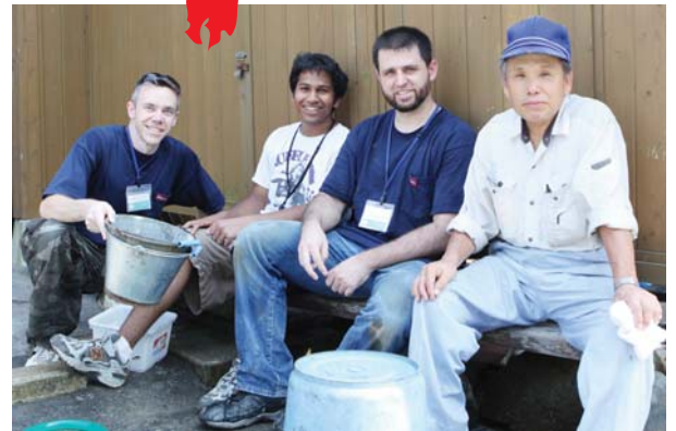
We spent a day tearing up wood flooring and mixing concrete to repair a foundation at a hotel in Kita Ibaraki.
